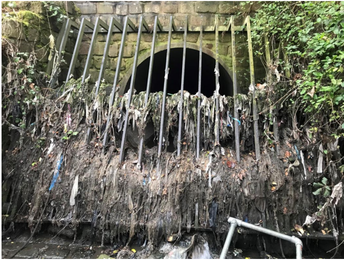
Fig. 2 An outfall from a CSO on the River Tame in Greater Manchester, UK. Figure reproduced with permission from ref. 25, Springer Nature Limited.
